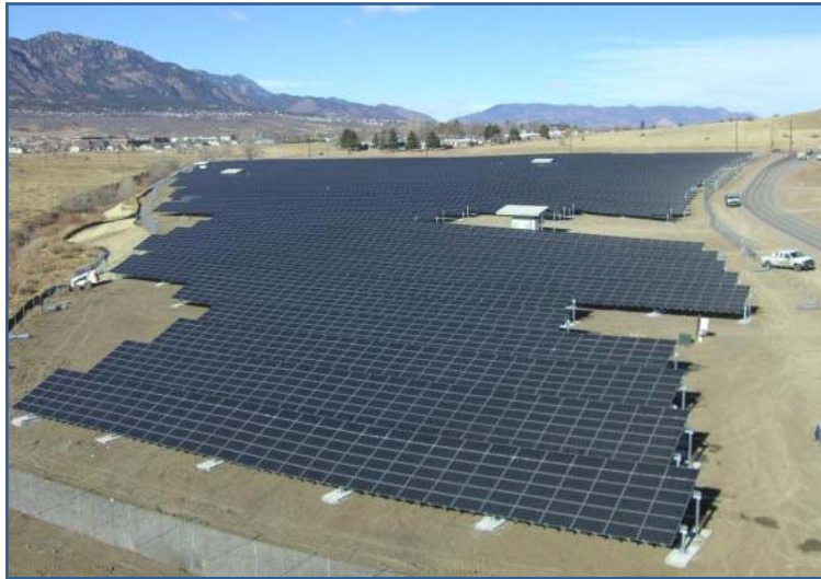
At Fort Carson, Colo., the Army partnered with a local energy provider in an enhanced-use lease. The energy provider built a photovoltaic solar array on top of a closed landfill. That site now provides energy to some 540 homes. U.S. Army photo.
